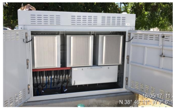
Figure 7 – In-line power regulators installed in the Uprgrid Portuguese demo site
