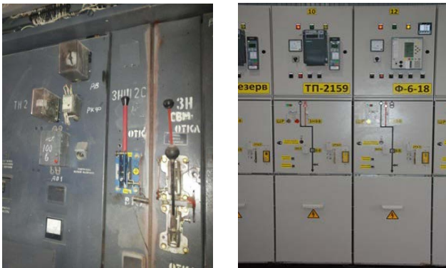
Old substation equipment New substation equipment Fig 4. Power grid renovation in pilot region.
