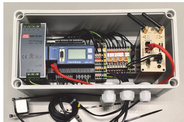
Fig. 2 – Measurement system built around a Janitza UMG 605 Power quality analyser.
