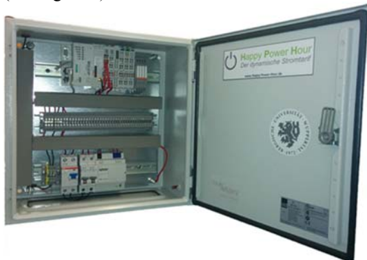
Figure 8: Developed automatization-system (HPH-Control-Box) for fully control of industrial processes
