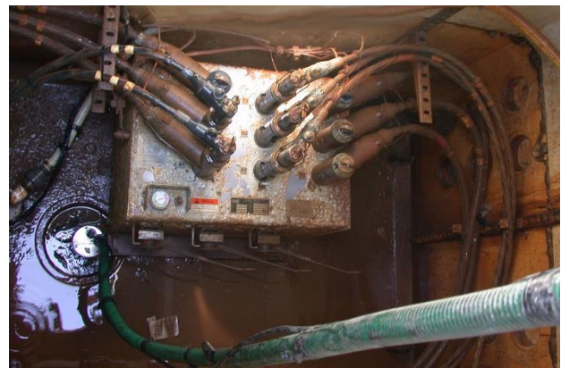
Figure 2. The same electrical vault as Figure 1, with the water pumped out
