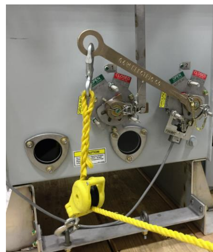
Figure 7. Switchgear Rope Rigging Example
