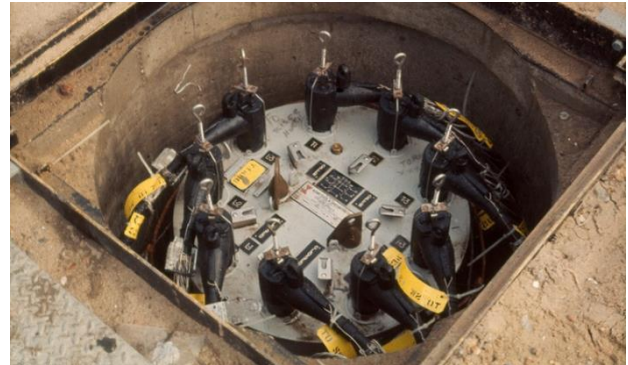
Figure 4. An example of a legacy vault designed for an oil switchgear, adapted for newer
