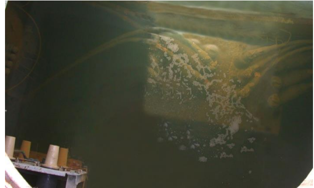
Figure 1. An electrical vault installation flooded with water
