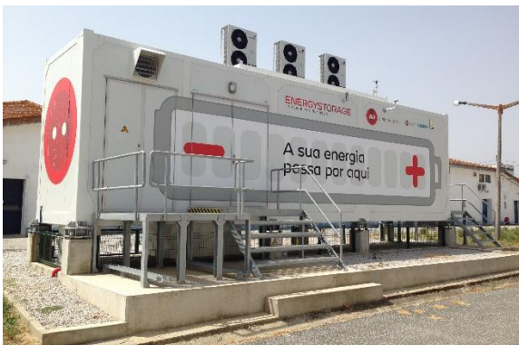
Figure 2 – EDP's ESS at Valverde, Évora.
