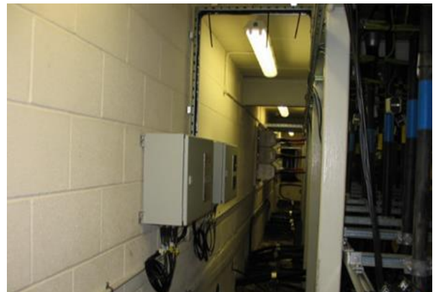
Figure 3 Node Units Installed at Belfast Central Main Substation
