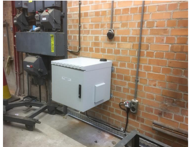
Figure 2 Hub Unit Installed Within IP54 Enclosure at Carnmoney Substation
