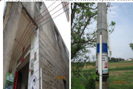
Fig. 8 Repeated Grounding Settings of TN System
