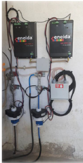
Figure 4 - Monitoring equipment installed in CNT 0024
