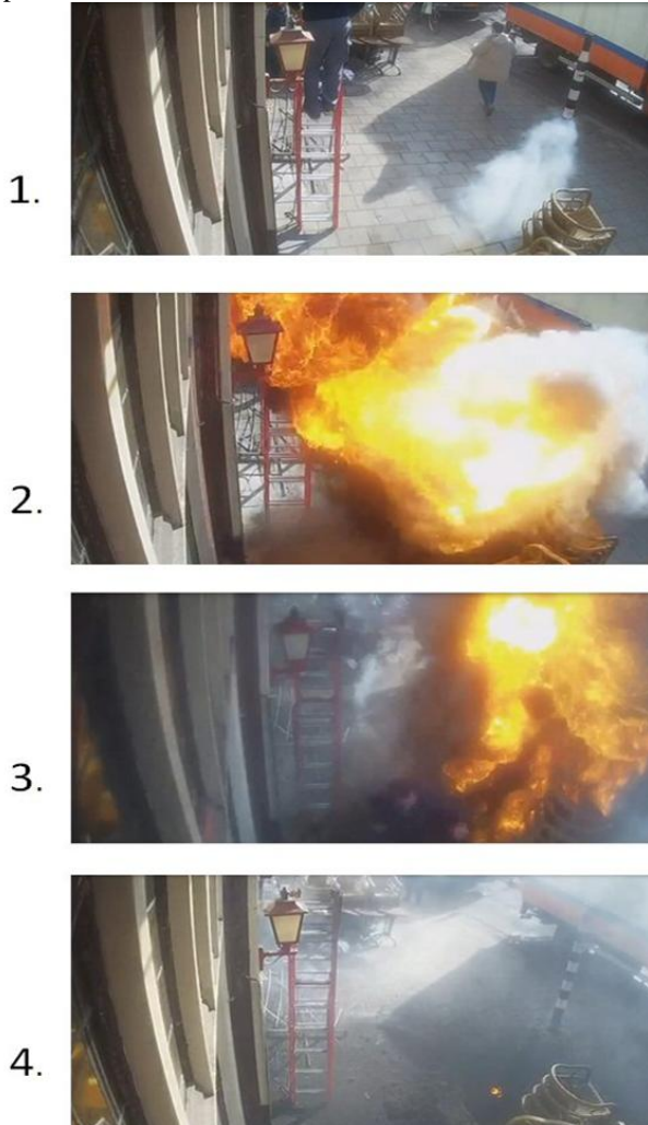
Figure 3: explosion of an oil filled MV Paper insulated cable joint below the pavement.
