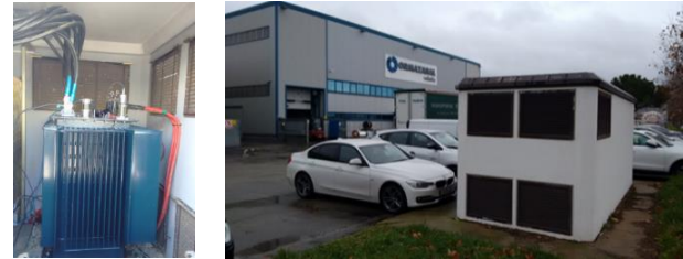
Figure 1. First smart distribution transformer in the field
