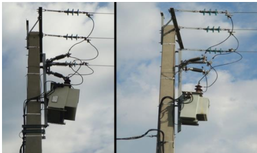
Figure 1: Typical Pole-top MV/LV transformer protected by three horizontal surge arresters.
