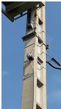
Figure 5: WSAM device installed on the earth cable.
