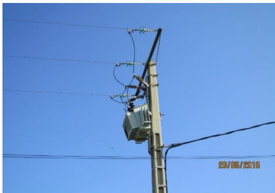
Figure 4: One of the targeted pole-top MV/LV transformer protected by three horizontal surge arresters.
