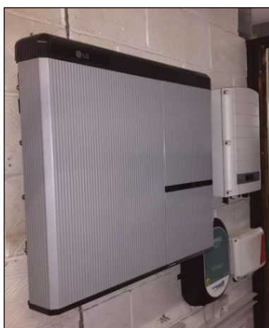
Figure 2: Example installation of battery energy storage, smart inverter and Domestic Load Controller devices in a customer's home
