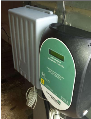
Figure 4: Example LV substation monitor
