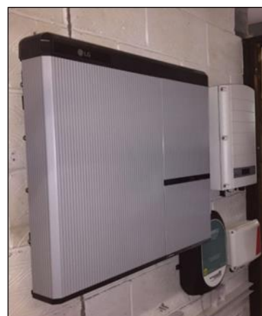
Figure 2: Example installation of battery energy storage, smart inverter and Domestic Load Controller devices in a customer's home
