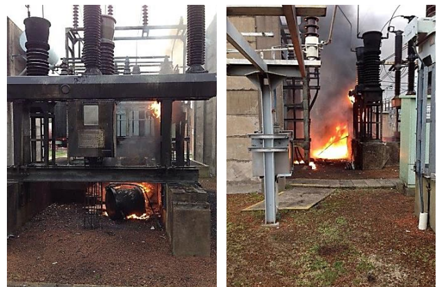
Fig. 2 - Failure with fire on a 132kV combined transformer.
