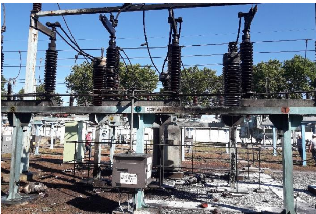
Fig. 3 - Failure on a 132kV current transformer damaging nearby equipment.
