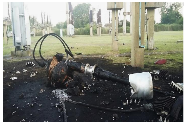
Fig. 1- Failure of a HV 220kV current transformer
