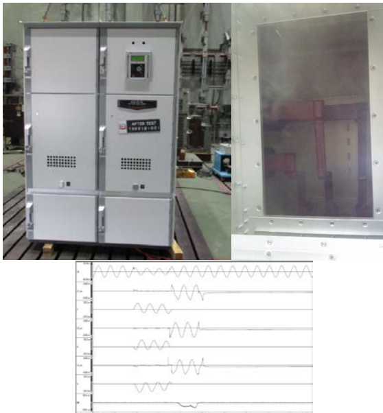
Figure 9 Internal arc test with actual panel and APS
