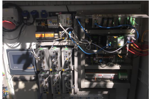
Figure 3: Photo of the installed hardware in a cable cabinet
