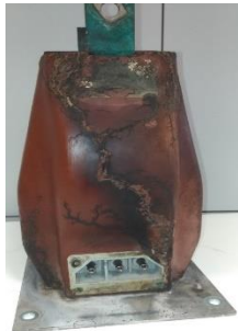
Fig. 12: measurement transformer identified as the source of the PD activity
