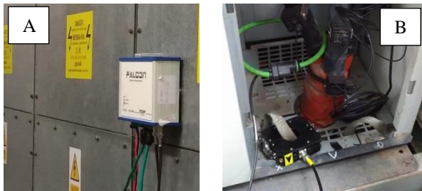
Fig. 5: installation of the PD detector (A) and the PD sensor (B) on a 15kV air insulated switchgear
