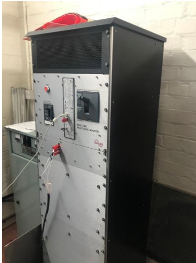
Figure 4 RTFLM Installed at Station View Primary
