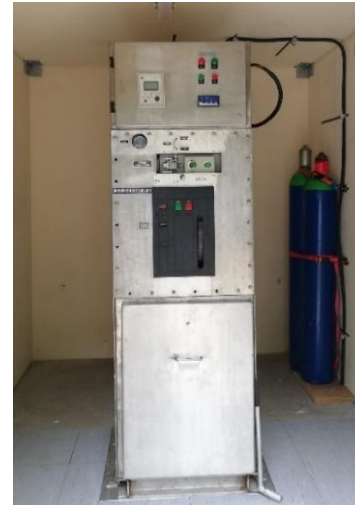
Figure 4: Pilot product based on dry air insulation inside a concrete building. (source: Westnetz GmbH)
