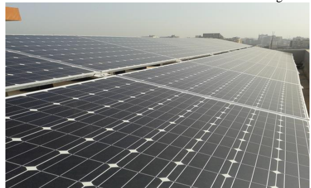
Fig.1 Photovoltaic Rooftop installed by NDEDC
