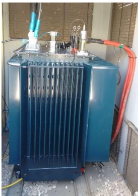
Figure 1. Smart transformer feeding Ormazabal Cotradis facilities 3
