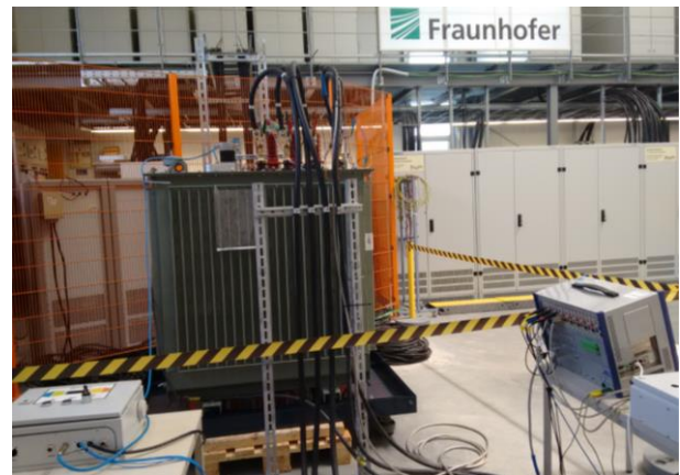
Figure 4. Smart transformer in the Test Bay.
